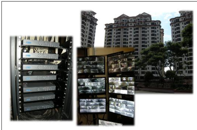
104 Cameras, 7 DVR Mawar Apartments in Gotong Jaya
